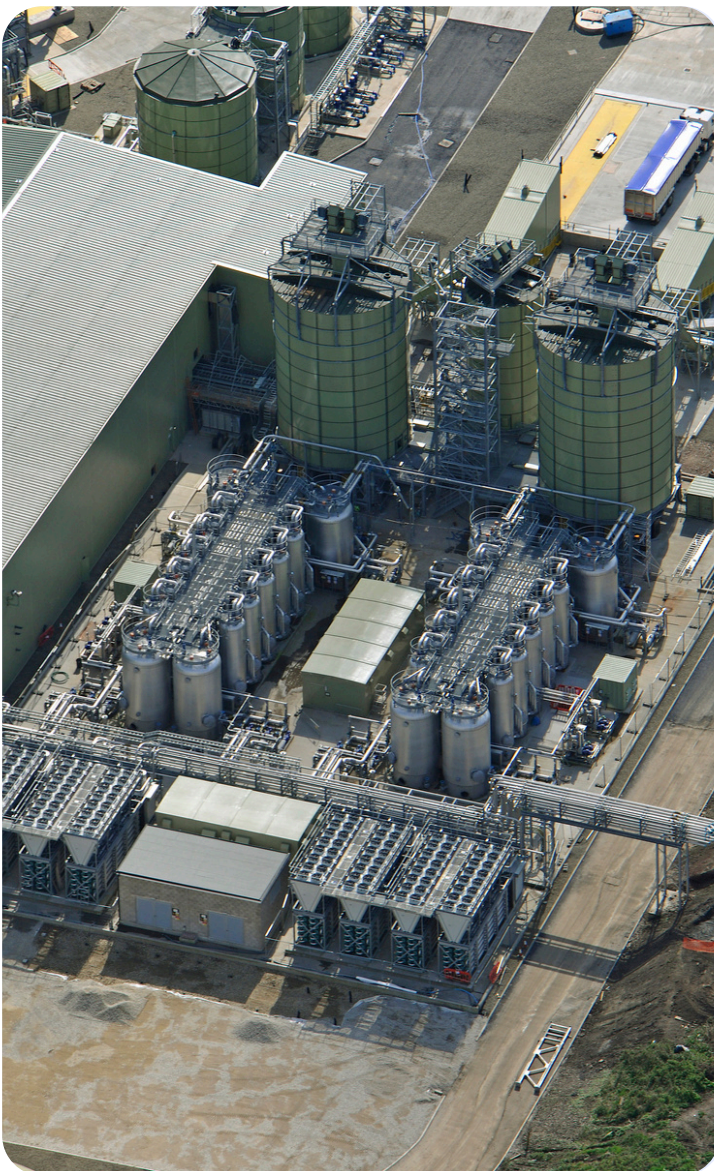
Cambi THP system at Davyhulme WWTP in Manchester, UK
