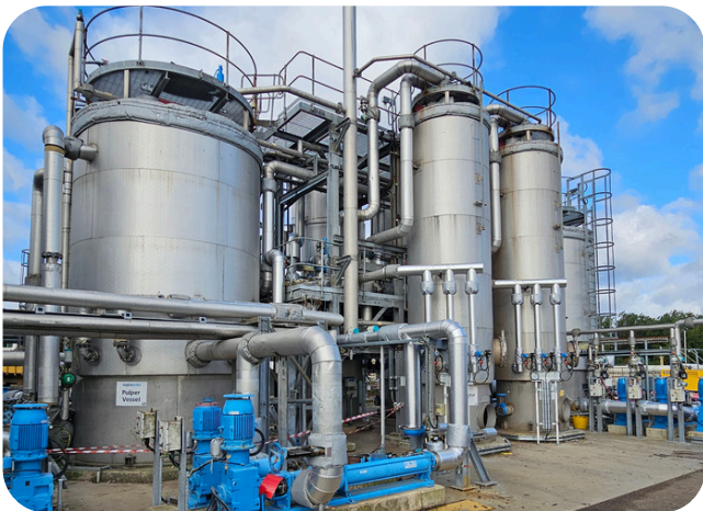
THP system upgraded for Anglian Water at the Whitlingham bioresources site in Norwich, UK
