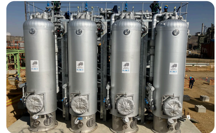
THP installed at Sasol's coal-to-liquids refinery in Secunda, South Africa
