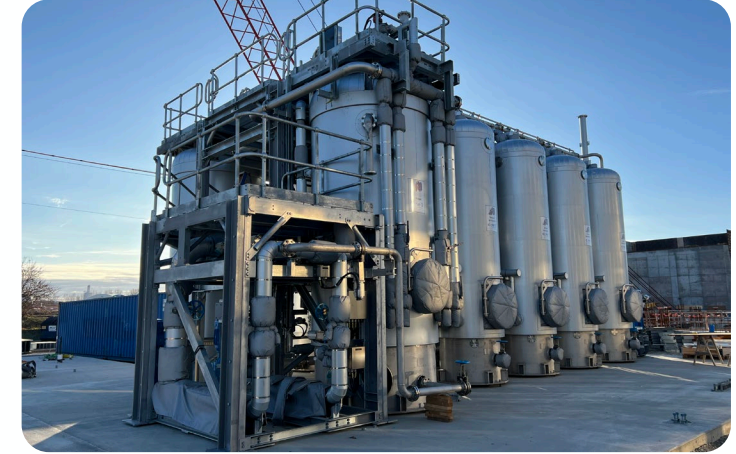
THP installed at Blue River wastewater treatment plant in Kansas City, Missouri, USA
